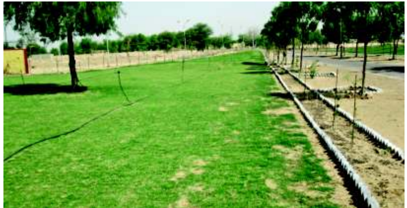
Micro sprinkler system for irrigation in newly developed lawn.
