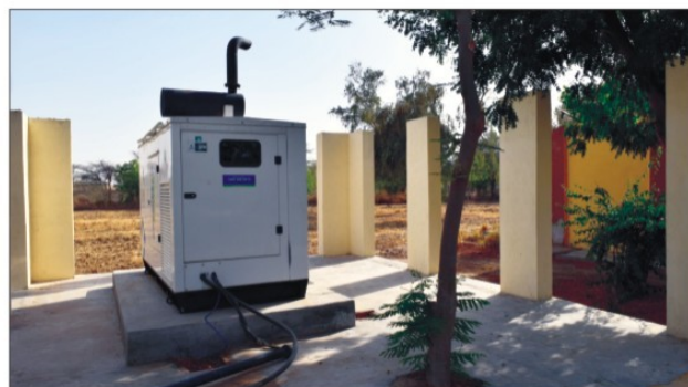
100 KVA Generator facility
